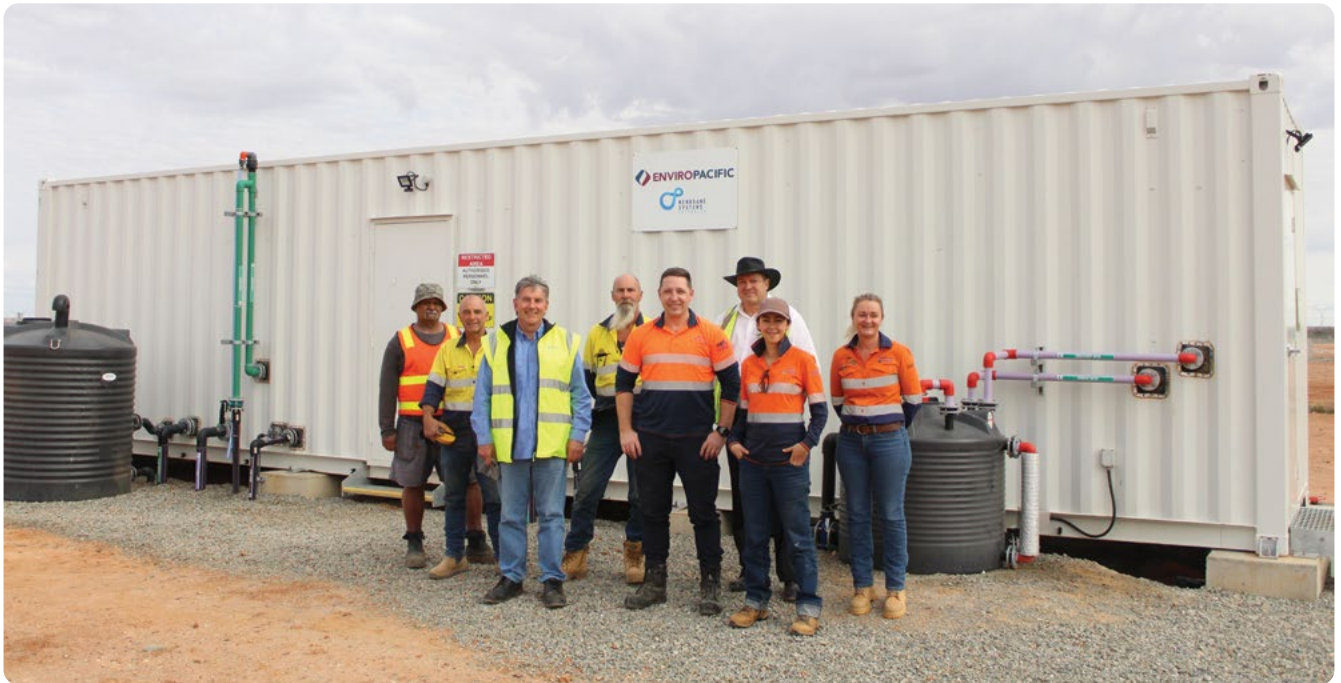
The Marla Desalination Plant is producing up to 87,000 litres of water each day.
