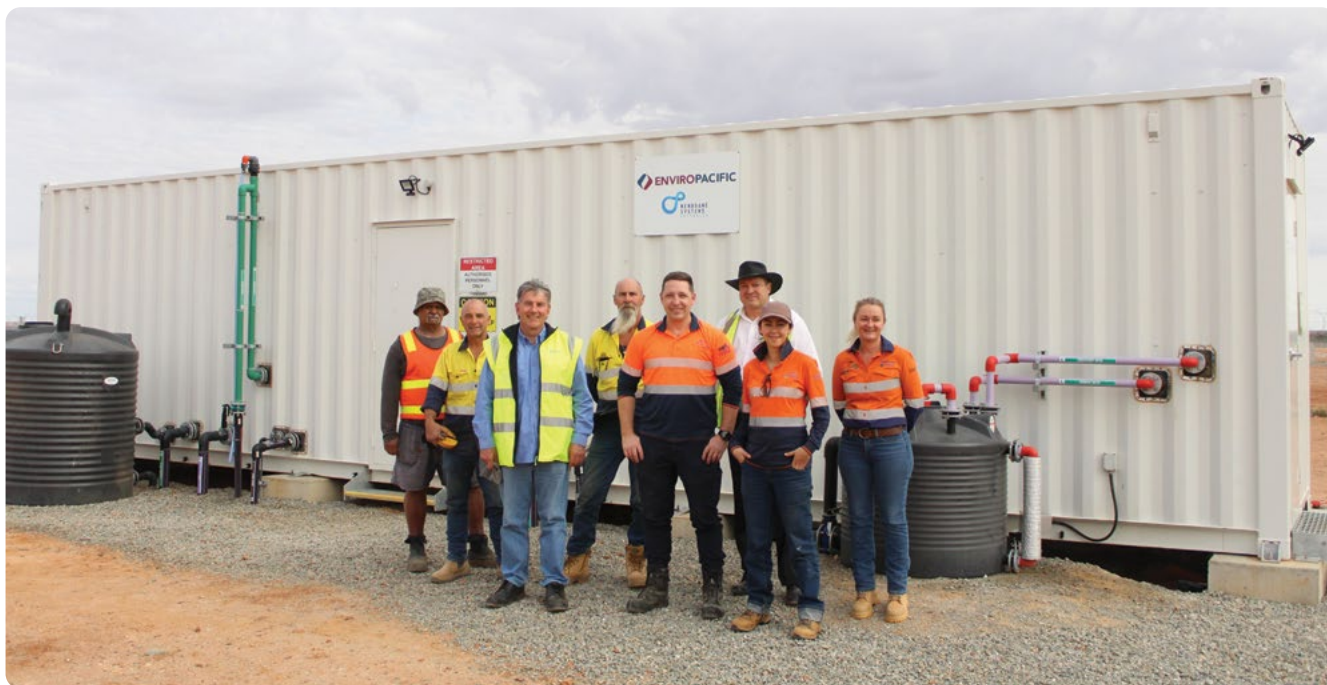
The Marla Desalination Plant is producing up to 87,000 litres of water each day.
