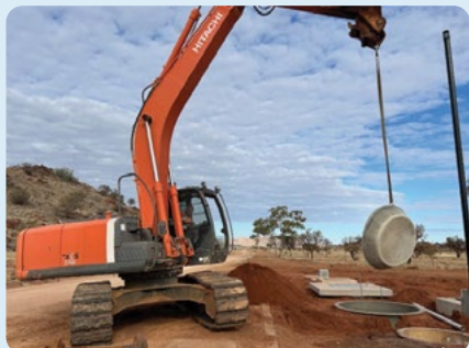
Upgraded wastewater infrastructure at Pipalyatjara in the Anangu Pitjantjatjara Yankunytjatjara Lands.
