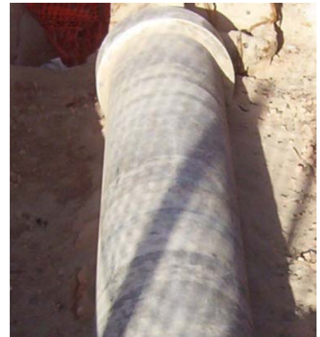
Photo 1: Asbestos cement pipe
