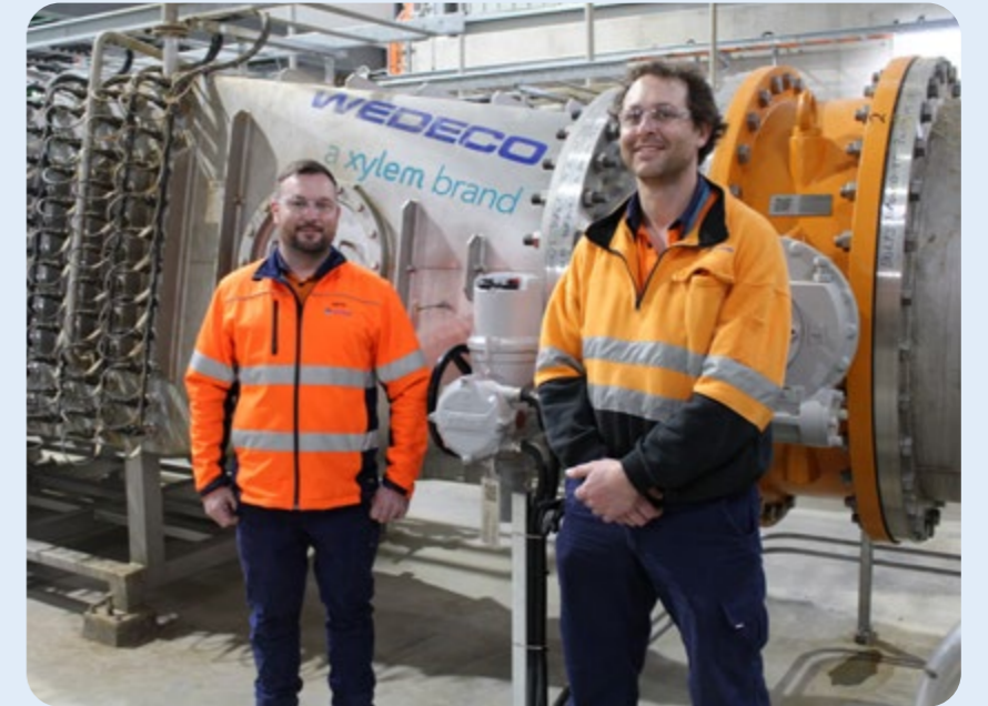
Project Coordinator David Flaherty and Plant Supervisor Ian Holmes at Happy Valley Water Treatment Plant with UV disinfection reactor.
