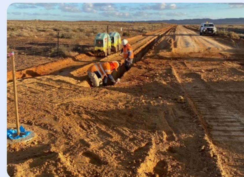
Workers from Aboriginal-owned recruitment service, RAW, replaced 22.5km of pipeline between Copley and Lyndhurst.
